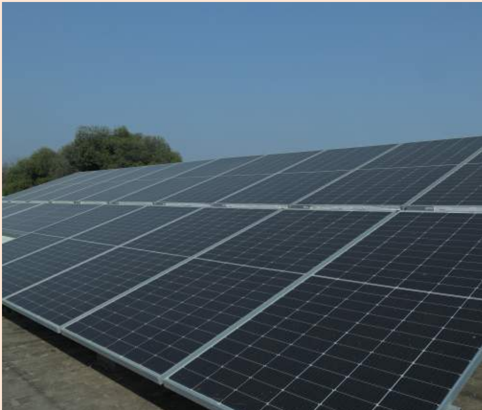
"Shining Bright: Harnessing Solar Power for Tomorrow!" Solar Panels-100 KVA"
